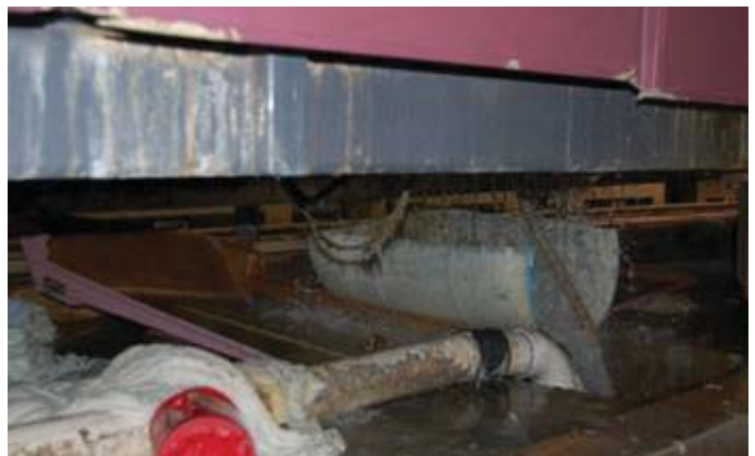
Water leaking from the seals under one of the tunnel washers cost the laundry operator 15-25 gpm from the worst seal.
