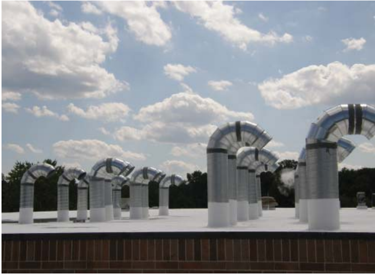
A view of a new intake and exhaust duct system for dryers in the plant
