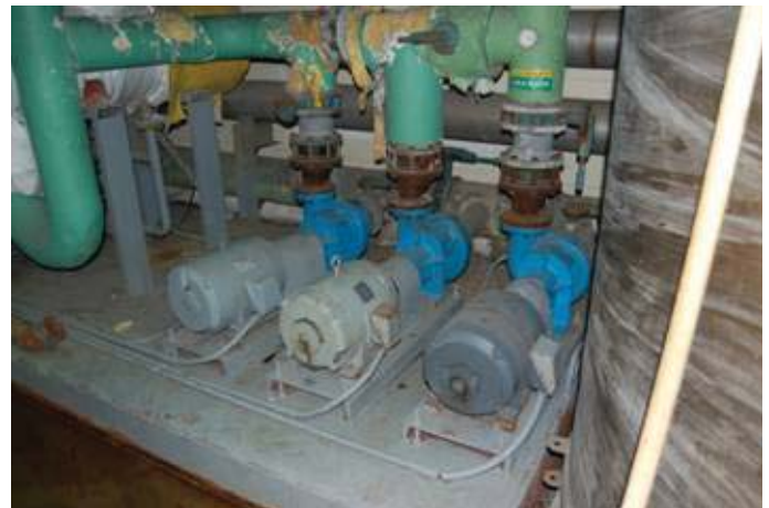
The existing plant's mechanical room was rife inefficiencies, including a boiler that operated at only 25-40% of full load, an inoperative wastewater heat recovery system and steam unit heaters that required complex maintenance.
