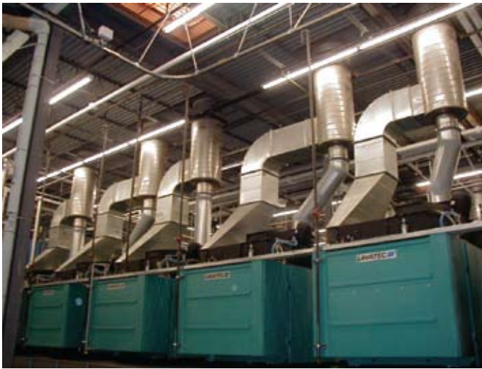
A view of dryers equipped with coaxial ducts
