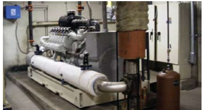
A view of cogeneration equipment
