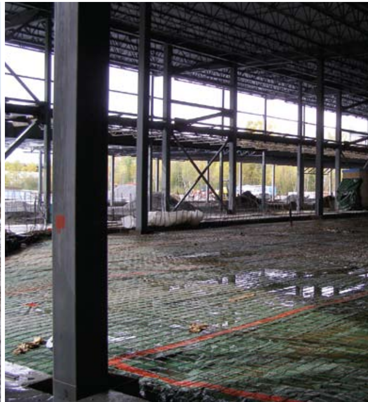
Construction moved forward in March/April 2006. Once the piles and beams were in place, builders added structural steel and the roof-support structure.
