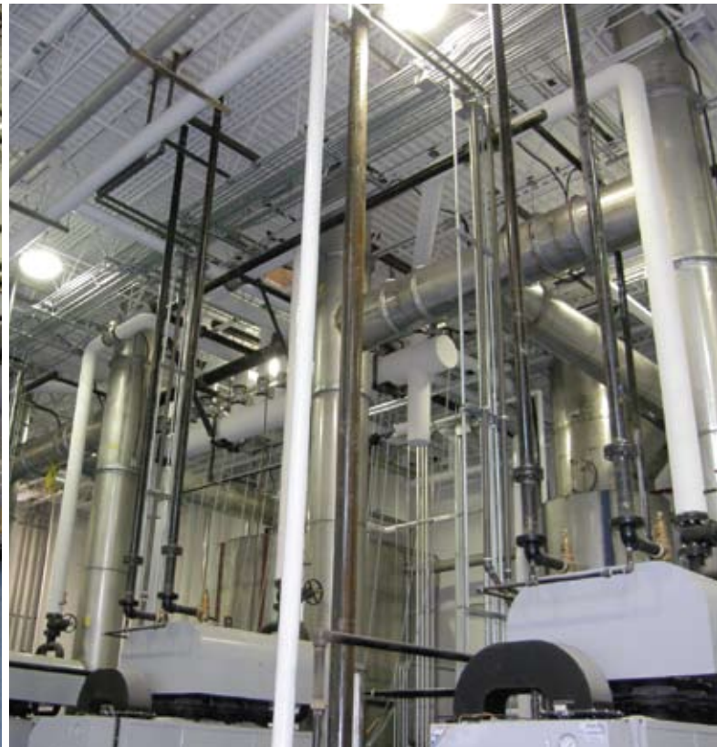
A view of pipes and ductwork leading from the top of the boilers to the plant's 26-foot ceiling.
