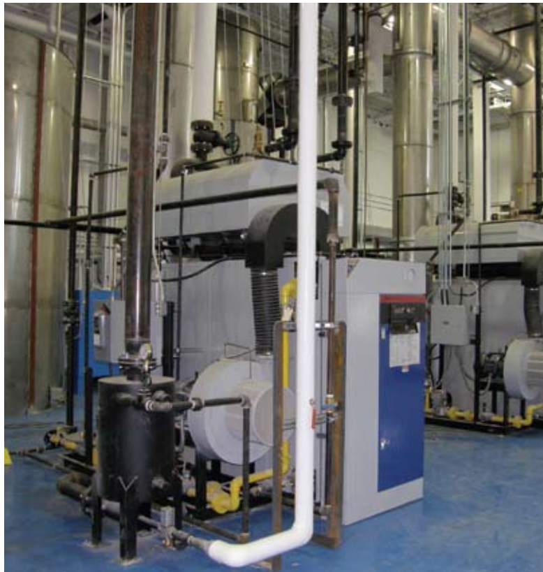
Above is one of four 300 BHP boilers in the plant. The plant also has a 100 BHP boiler for sterilization of OR packs.
