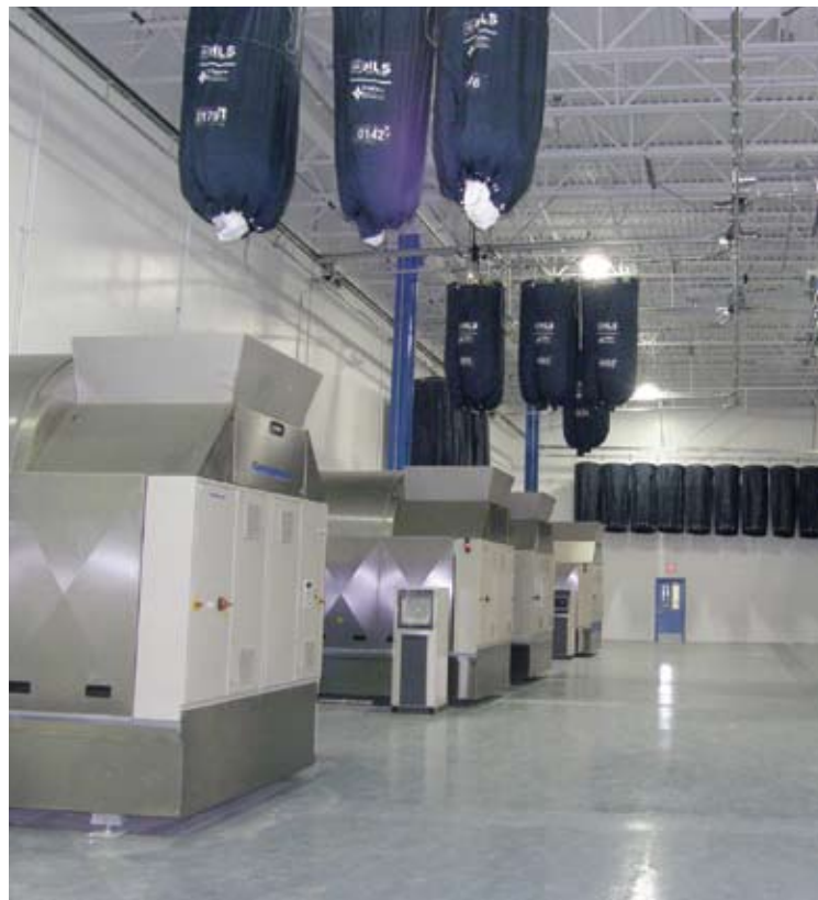
A view of the plant's four tunnel washers located in the "mezzanine/equipment platform" area. These tunnels feed clean goods to 24 dryers.
