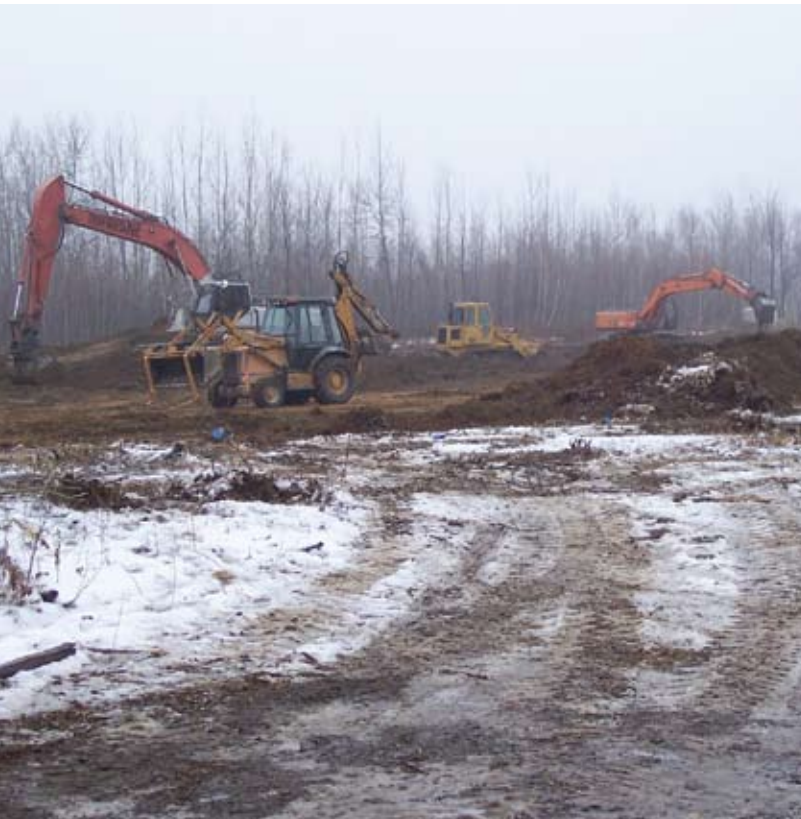
Due to wet conditions at the site, contractors drove more than 200 steel piles down 75 feet to bedrock formations in order to secure the foundation of the new plant.
