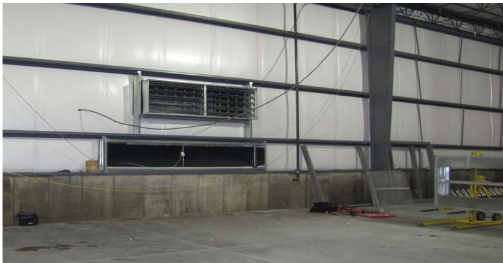
The photo above shows part of the air/hvac system, providing positive to negative airflow. This will ensure compliance with Healthcare Laundry Accreditation Council (HLAC) standards for a healthcare facility.
